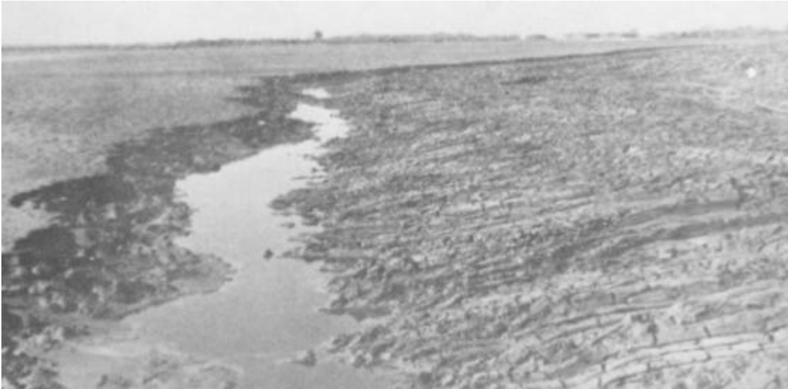
Figure 5-11. Construction of ditch 12 to 18 inches deep with excavated material cast on interior slope of perimeter dike
