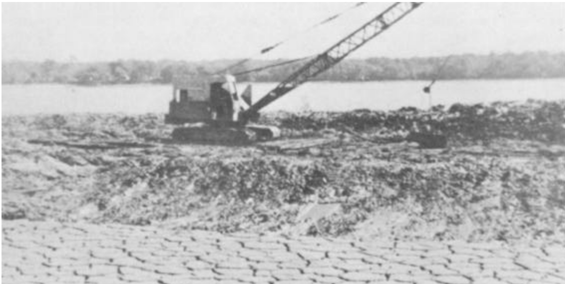
Figure 5-10. Small dragline on mats working on berm deepens shallow perimeter drainage trench
